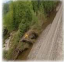
Before: Erosion at Base of Bank Protection
