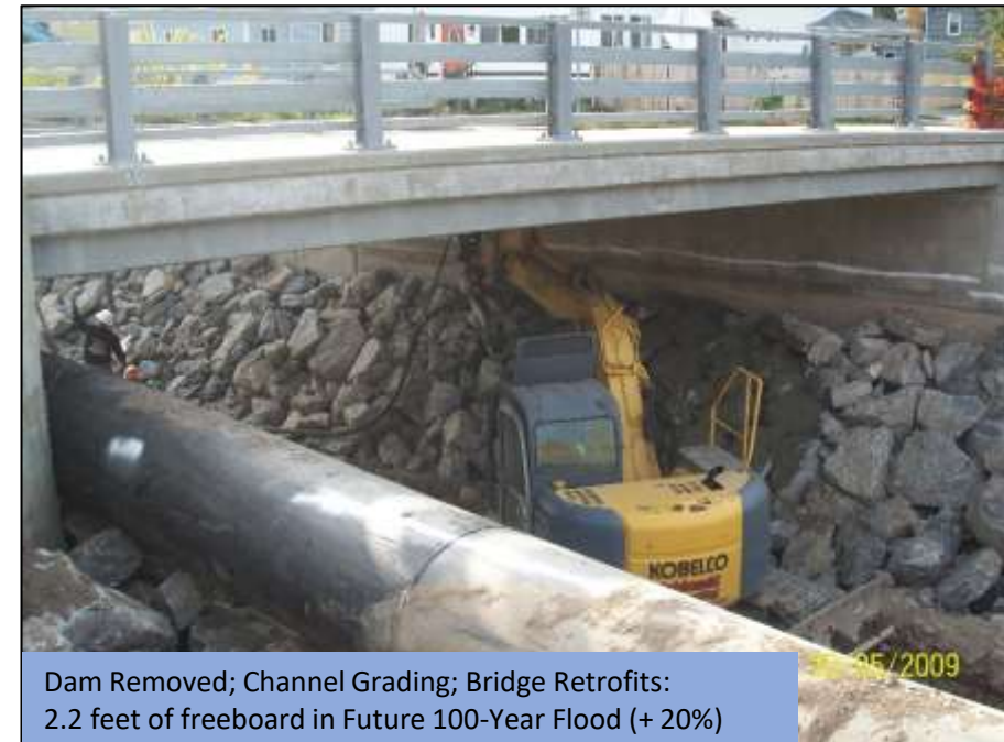
Frederick St Bridge Pre-Project: Overtopped in < 10-Year Flood
