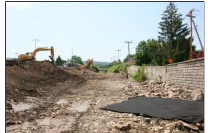
Top: Remington Arms Dam, Ilion, NY, before construction, 2019 Middle: During construction, 2020 Bottom: During construction, 2021
