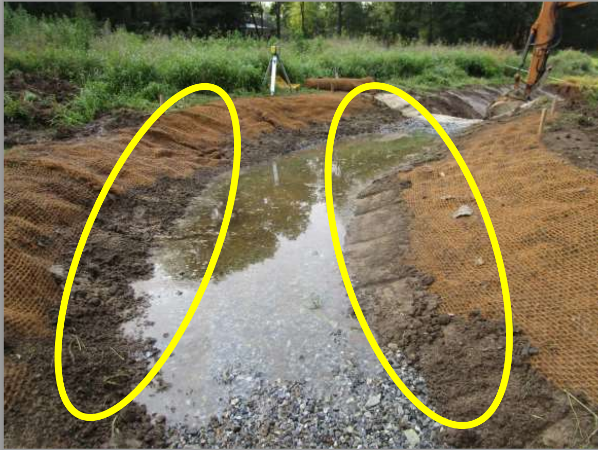
Missing stakes along channel reach 2
