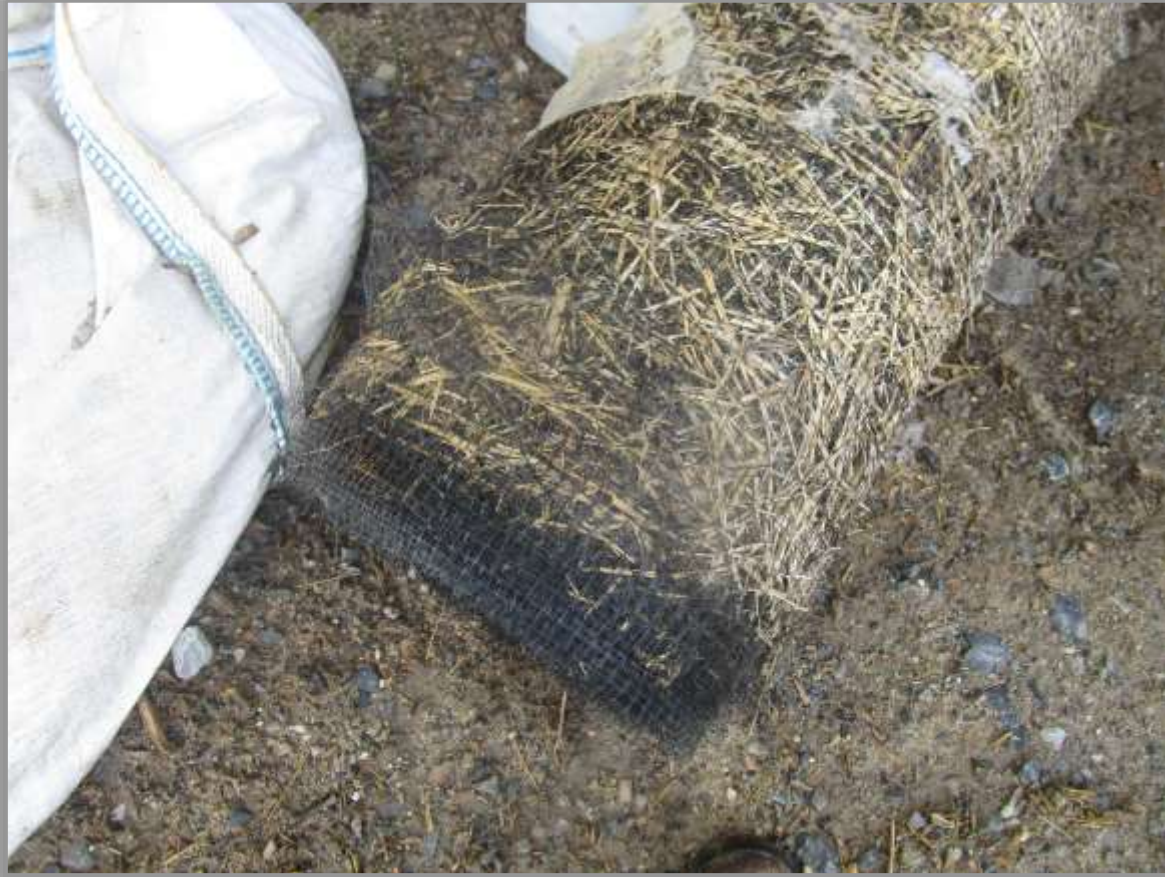
Incorrect materials brought on site
