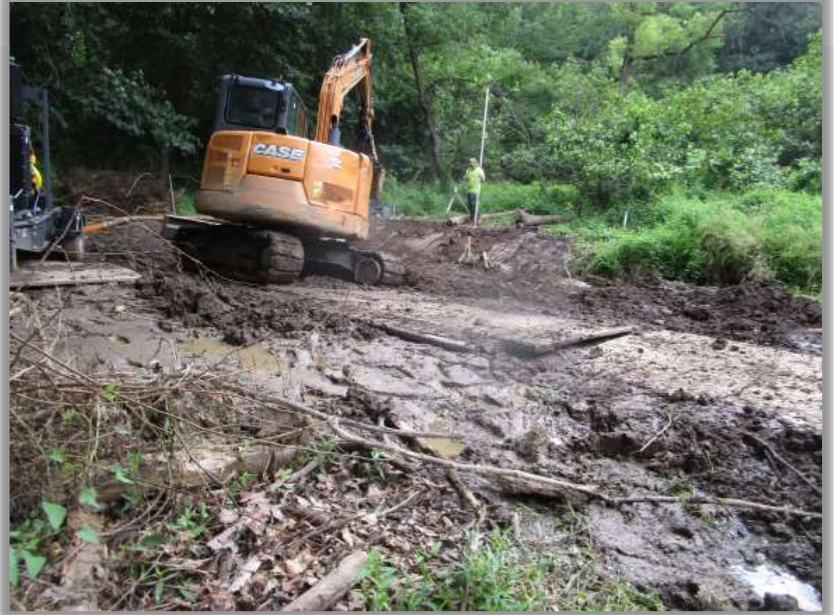
Inexperience working in saturated soils
