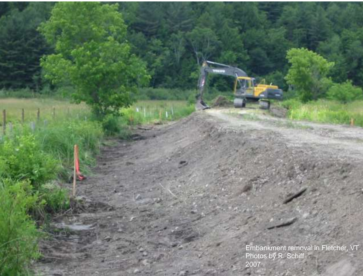
Railroad Embankment Disconnecting Floodplain
