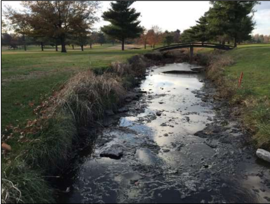
Upper reach of was overwidened, cut down to bedrock with eroding banks.
