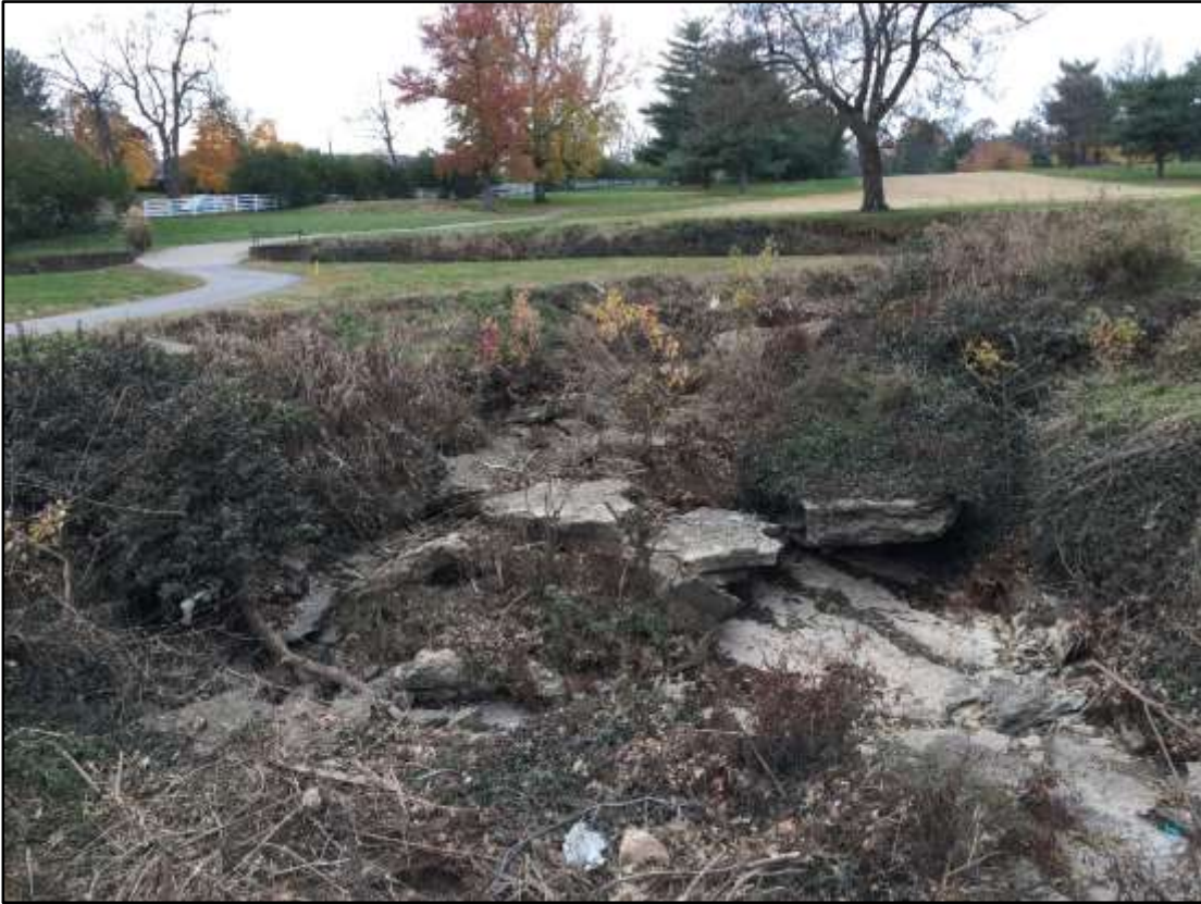
Lower reach was severely incised and had downcut to bedrock.
