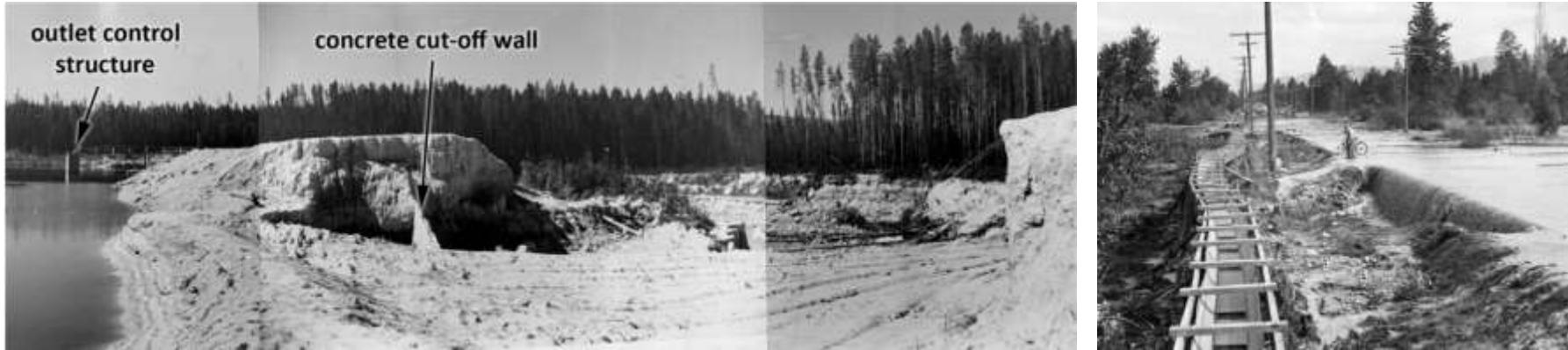
May 1941 – 36 m breach of EC No. 4 Dam
